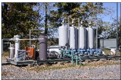
Molecular Gate system at a facility in Southern Illinois
