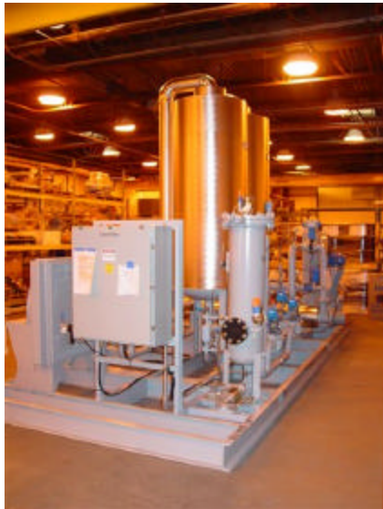
Natural Gas Dehydration Unit
