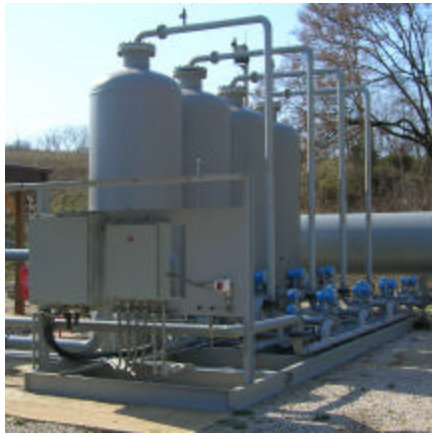
Natural Gas Treatment Unit
