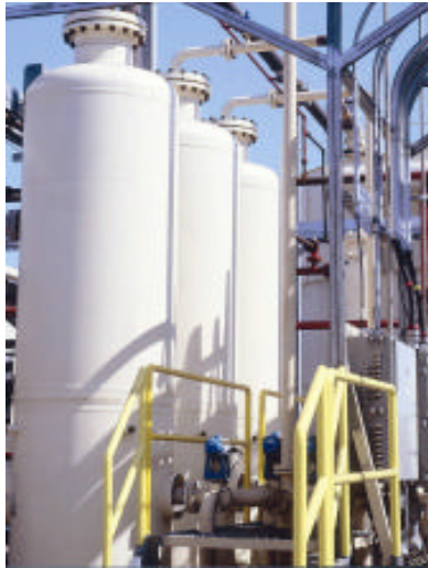
Molecular Gate ® System at the Tideland Facility in Long Beach
